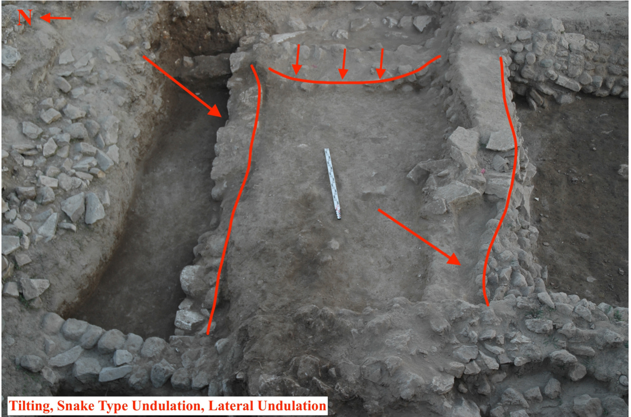
Figure 8. Western view of the tilting, snake-type undulation, and lateral undulations of the walls in the front room of House-2, belonging to the Liman Tepe VI-1b phase (Photograph: Dr. Ümit Gündoğan, IRERP Archive).
