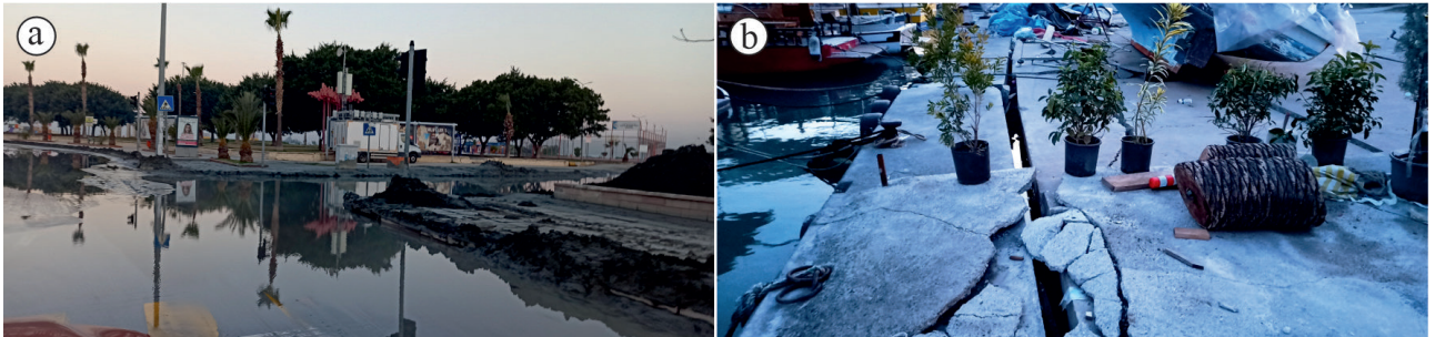
Figure 8. a) Local puddle and liquefaction-related silt heaps on the road 6 days after the earthquake. b) Cracking in the fishery port due to the splitting and settlement of the coastal fill. Standing greens indicate that seawater has not come from the sea to the shore. Image locations are indicated in Figure 3.
