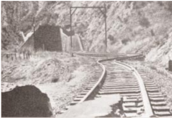
Figure 2. Kern County urban railway tunnel. A view from the entrance of the tunnel showing bent rails near a zone of intense fracturing along the White Wolf Fault. Source: SCECDC 2002.
