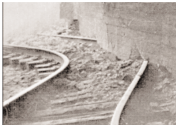
Figure 3. Bent rails inside the Kern County urban railway tunnel. The White Wolf Fault had a both compressive and lateral dislocation during the 1952 Kern County earthquake. Indicative of this type of fault dislocation is the fact that the rails are bent and continuous underneath the tunnel wall, showing that the wall was lifted up enough for the rail to slide underneath. Source: SCECDC 2002.
