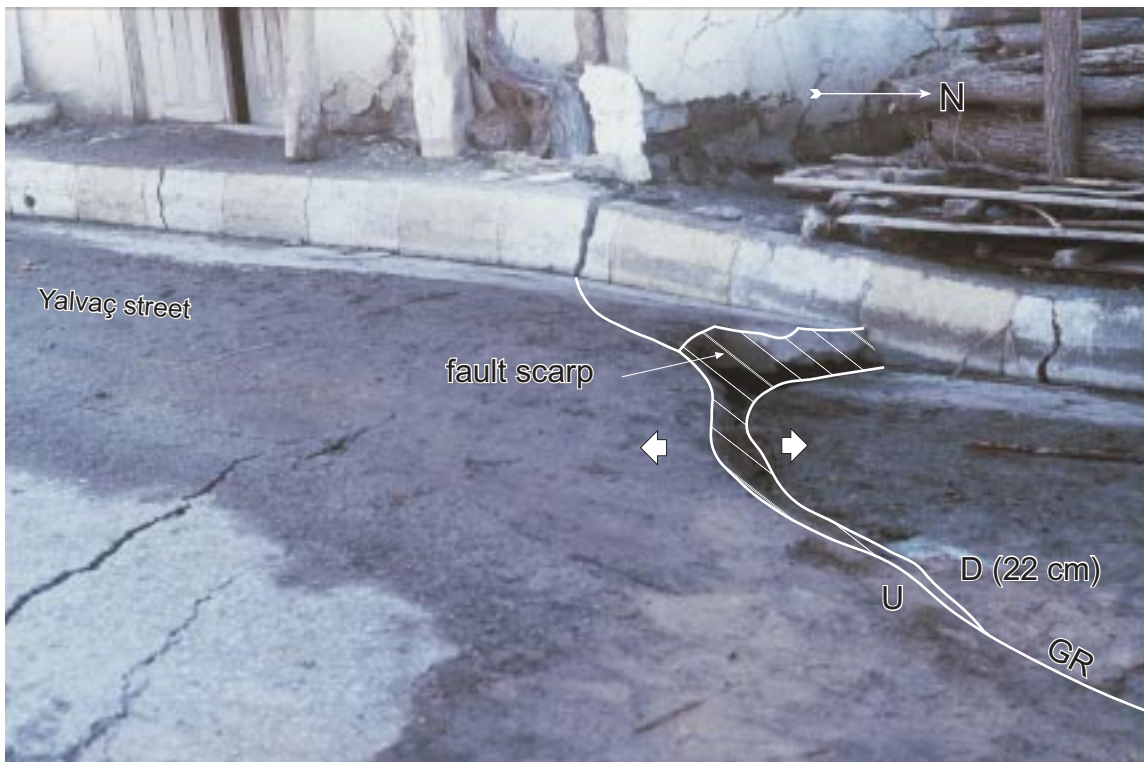
Figure 15. General view of the Çay ground rupture that cut the NNW-trending asphaltic Yalvaç street and down-dropped it as much as 22 cm (view towards west). U– up-thrown block and D– down-dropped block (hanging-wall block).
